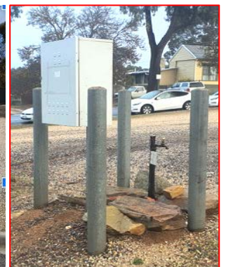
Figure 8: Power box and tap
