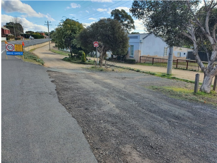
Figure 23: Poor state of access from Duke Street
